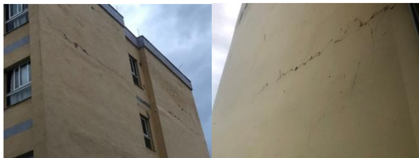
Figure 2. Building hit by an earthquake in Shijak, Albania, in 2019.
