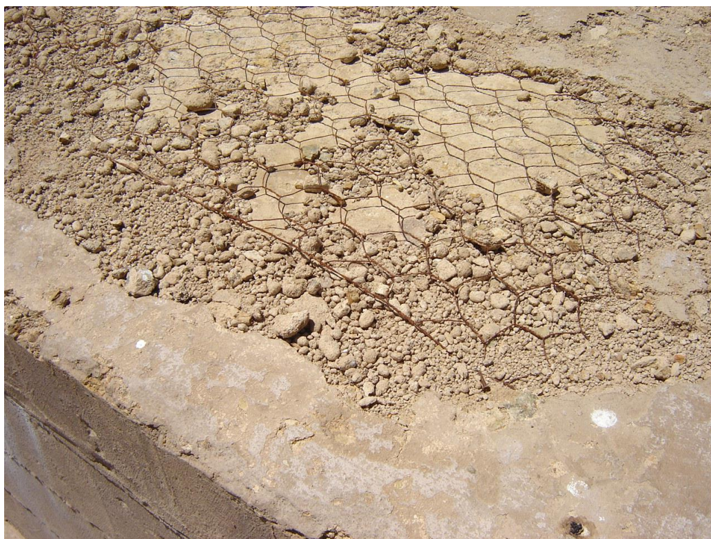
Figure 11. Detail of incompatibility of materials in an intervention for conservation of a rammed earth fortification, causing damage in the structure.
