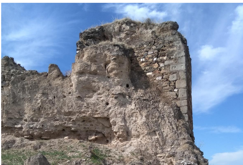
Figure 9. Action of water and structural failure in a military rammed earth structure (Juromenha, Portugal).
