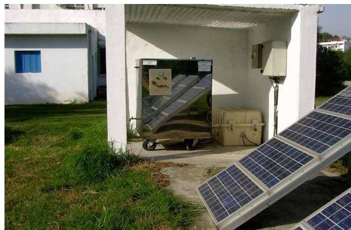
Figure 4. External view of the water treatment pilot unit.
