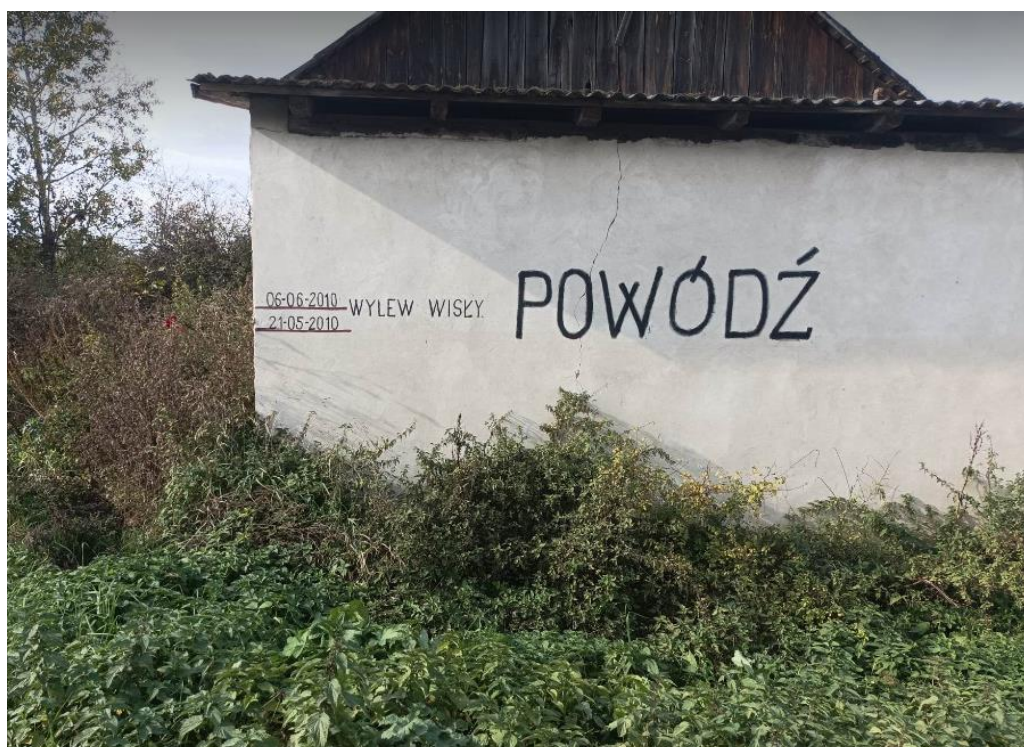
Figure 16. Flood mark on a private house in the Kłodnica settlement. Photo: Daria Krasiewicz, October 2022. In Polish: wylew Wisły - inundation from the Vistula River; powódź – flood. Location available at: http://openhydrology.org/maps/flood_mark/?zoom=17&lat=51.233081&lon=21.876681 , cf. [68].
