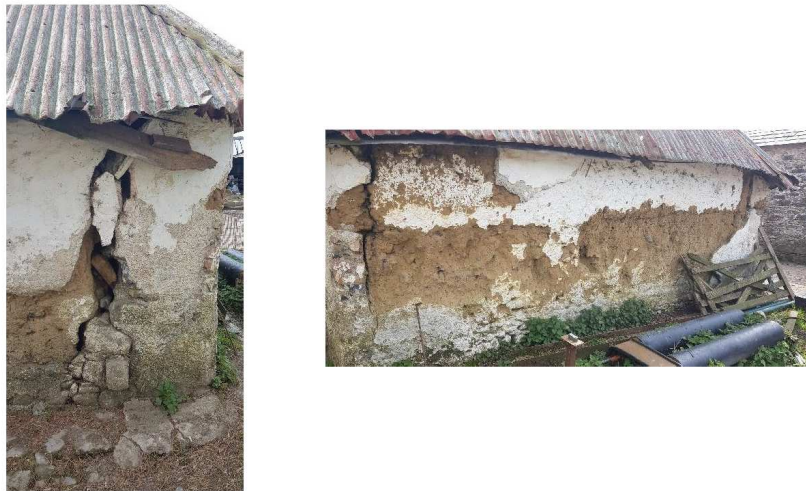
Figure 3. Vertical cracks in a cob building located in County Kildare, Ireland (pay special attention to the cracks at the corners running all along the wall's height).
