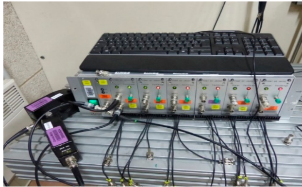
Figure 5. Somelec Wheatstone bridge and calibrated Rogowski coils on different cables.
