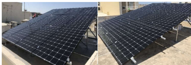
Figure 4: (a) PV System in Fgura, (b) PV system in Tarxien
