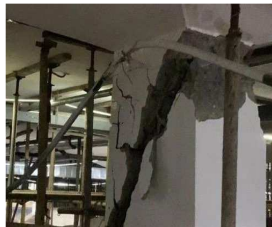
(b) Damage of column elements
