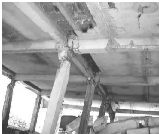
(a) Damage of joint elements
