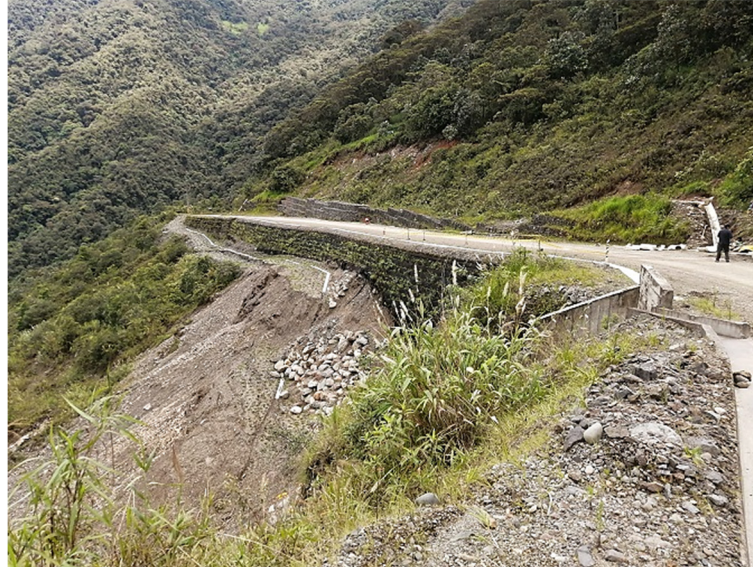
Figure 2. A view of the middle part of the landslide area where the road was affected (cut) and reconstructed, applying observed earth-walls. In this location, the movement is prone to continue at a low displacement tax. It can be observed the high slope on the landscape.
