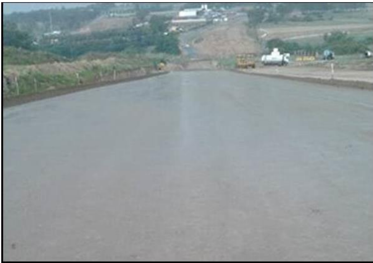
Figure 19. One week after placement of base with no protective later added – 200 mm of rain with installed curbs acting as a channel
