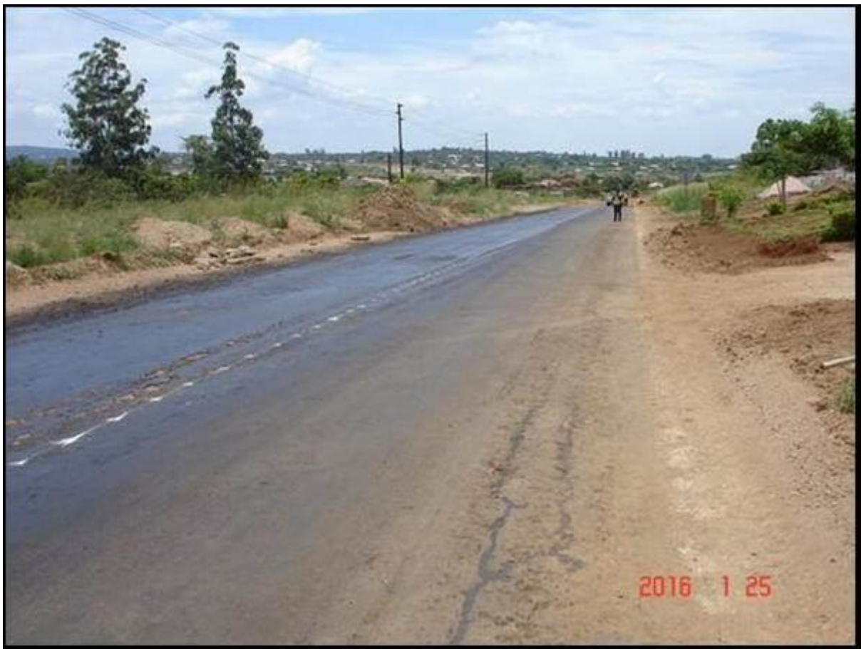
Figure 30. Condition of the base with prime after two months of trafficking during the summer holidays and applying of a tack-coat before surfacing
