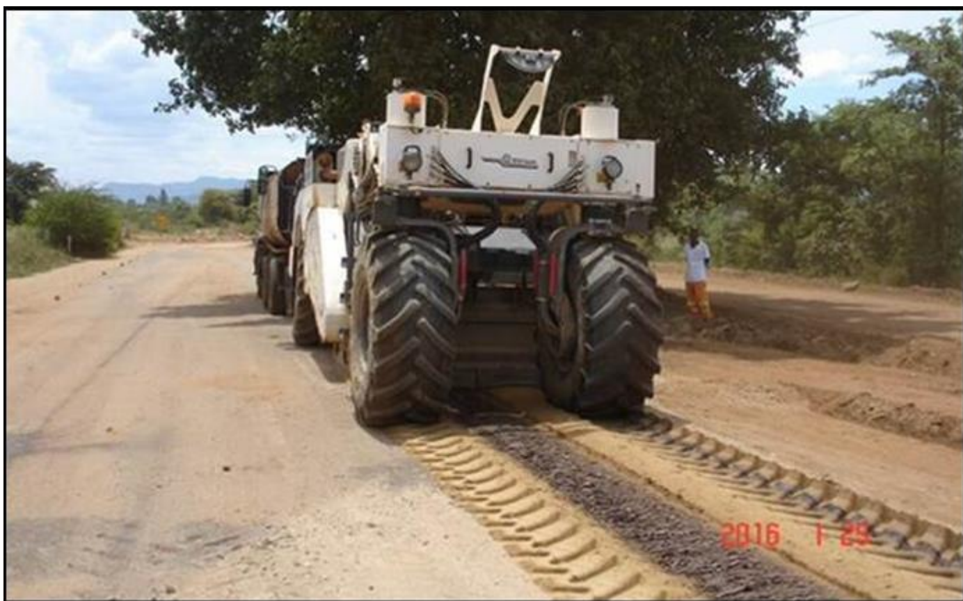
Figure 59. Uneven distribution of the stabilising agent behind the recycler caused by blocked spray-nozzles
