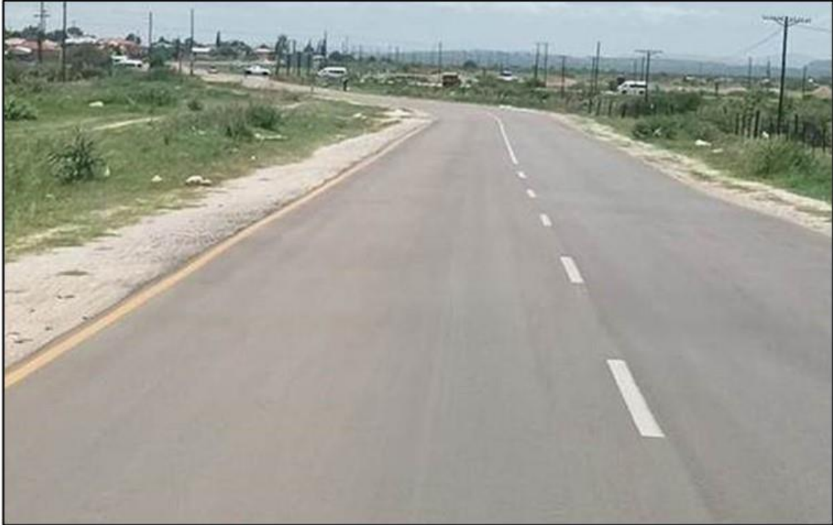
Figure 46. Condition of the surfaced road 6 years after completion
