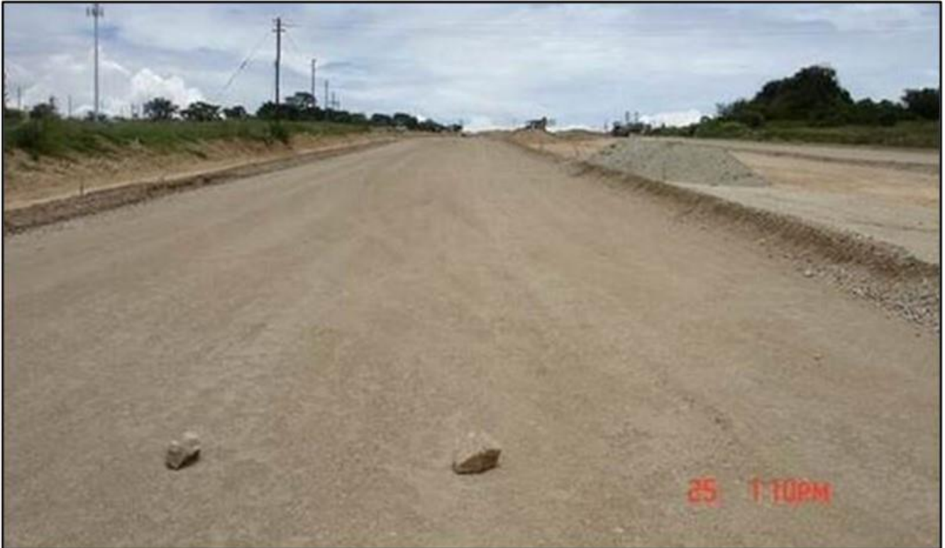
Figure 40. Condition of the sub-base after being subjected to the rain
